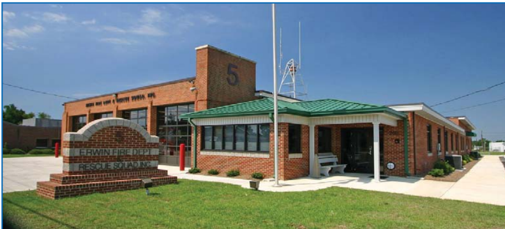
“The Erwin Fire Station renovation required construction staging in order for vehicle bays to remain operational.”
